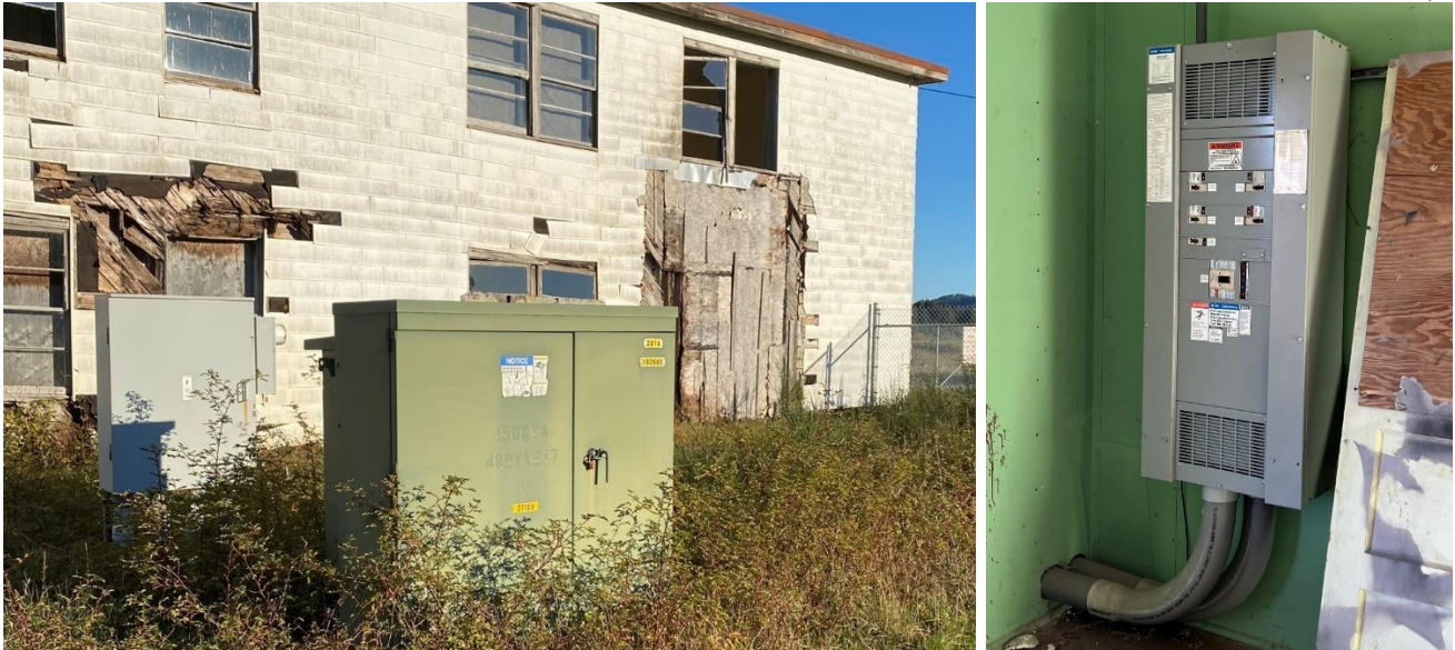
Figure 7: Hangar main transformer [left] and main distribution panelboard [right]
